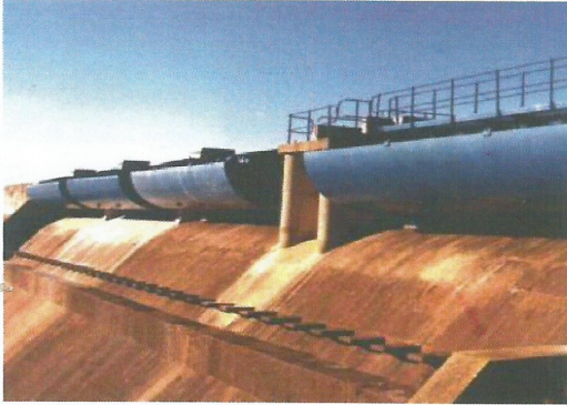
Raising of the Belfast dam using TOPS spillway gates to increase storage capacity by 50 %
