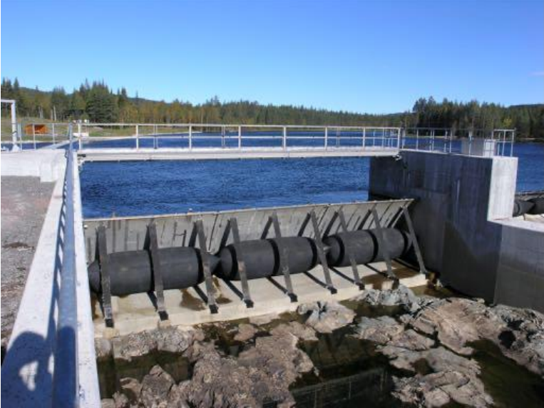
Figure 2 Flap gate supported by airbags.
