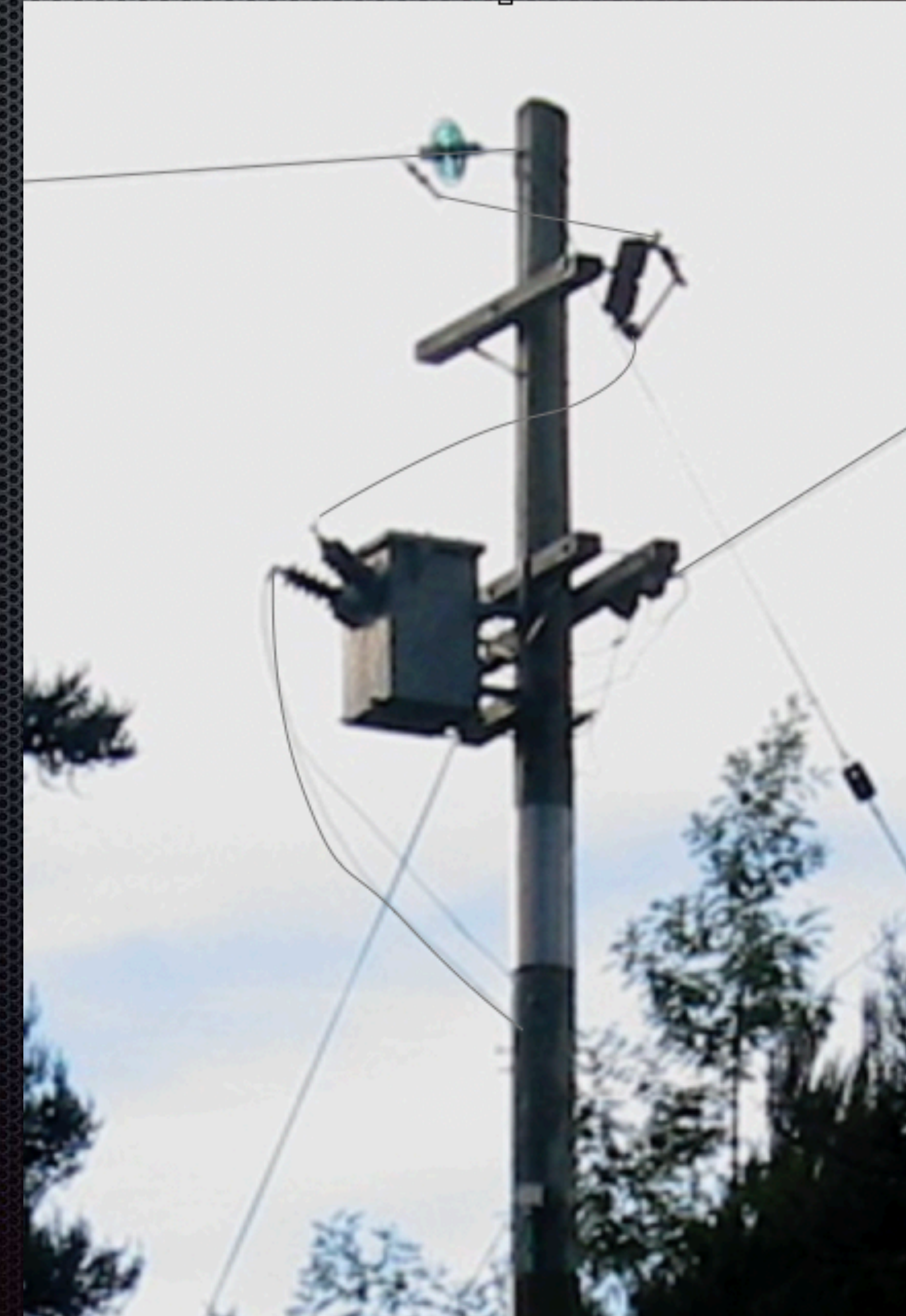
NZ SWER transformer
