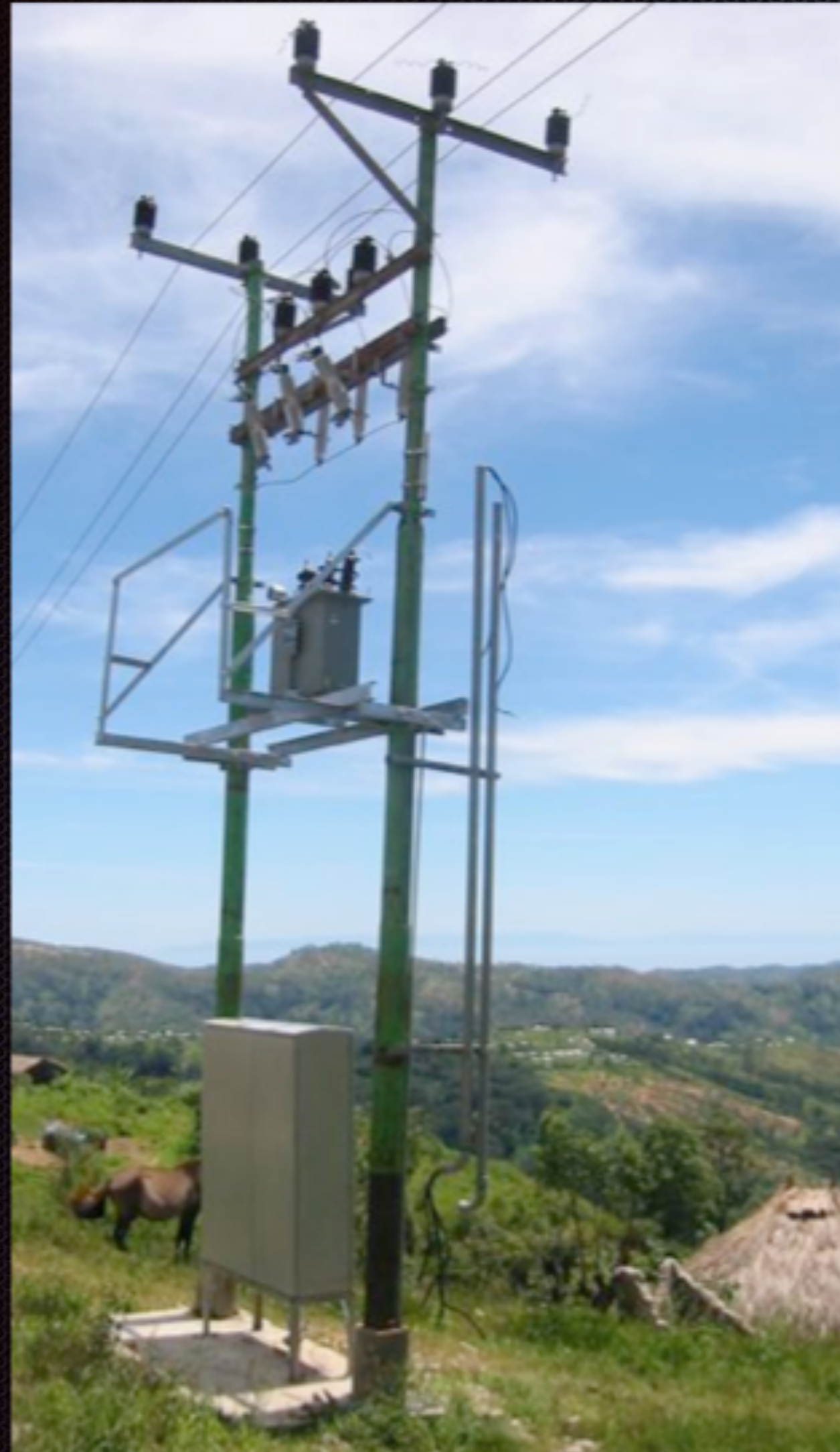
Transformer in E Timor
