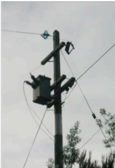
16 kVA SWER transformer
