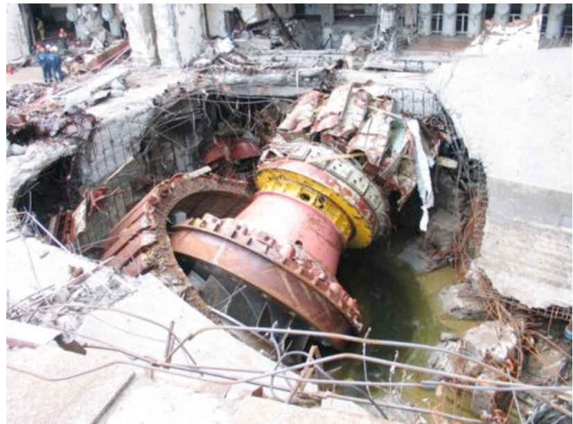
Figure 4 Unit 2 turbine and rotor spider
