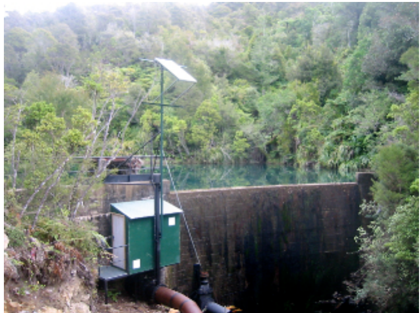
Dam, intake and solar cell
